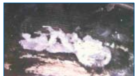
Figure 3. Corrosion of a Zeron 100 flange caused by the use of a graphite-filled gasket.
